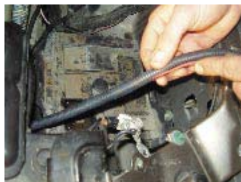
119. Run supplied 22 gauge wire through firewall harness boot to fuse #18 and connect using supplied fuse tap making sure to solder all connections, then cover wire with loom, but do not allow wire to scuff on body around boot (use supplied fuses)
