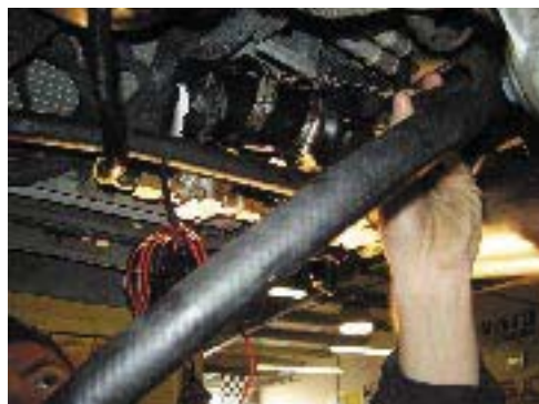
115. Extend intercooler pump wire using supplied splices, wire, and plug in, making sure to use solder and shrink wrap on all connections.
