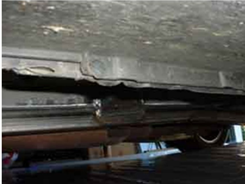
The image above shows the welded subframe connector on the front frame rail.
